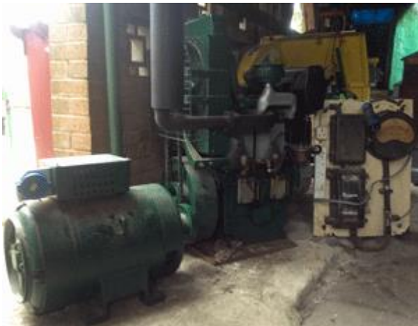
1951 Petter 2 Cylinder 10HP Diesel Engine Generator Control Switch Board & Base
